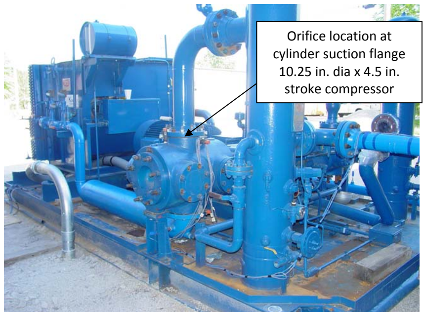
Fig. 5: Closed loop test compressor showing orifice location
