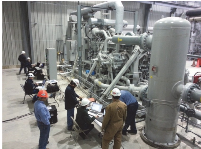
Figure 9: First PAN™ Manifold unit undergoing extensive thermodynamic performance testing.
