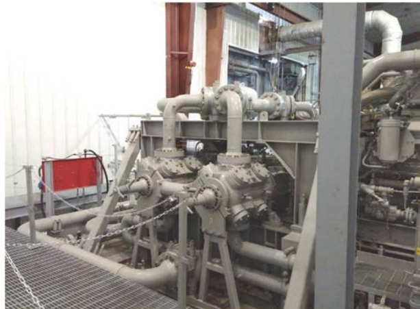
Figure 12: Second PAN Manifold unit installed (with work platforms) – right side view
