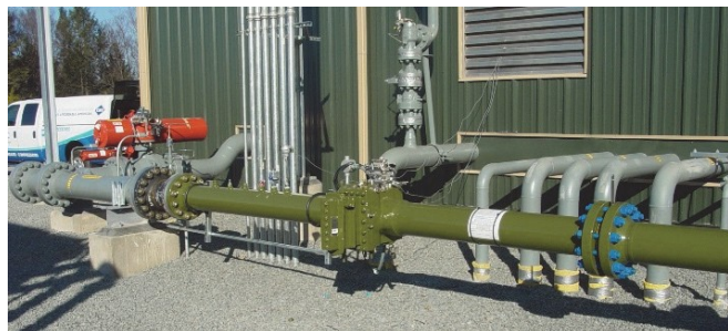
Figure 10: AGA flow meter in suction line to PAN™ Manifold unit, used for performance testing.
